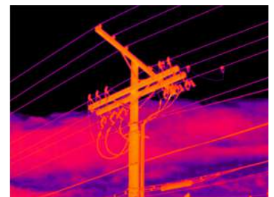
Electrical connection of transmission tower
