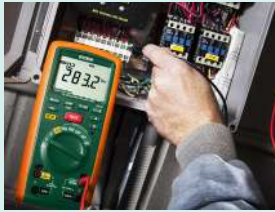
Voltage check on motor starter
