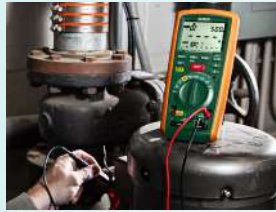
Insulation test on pump motor
